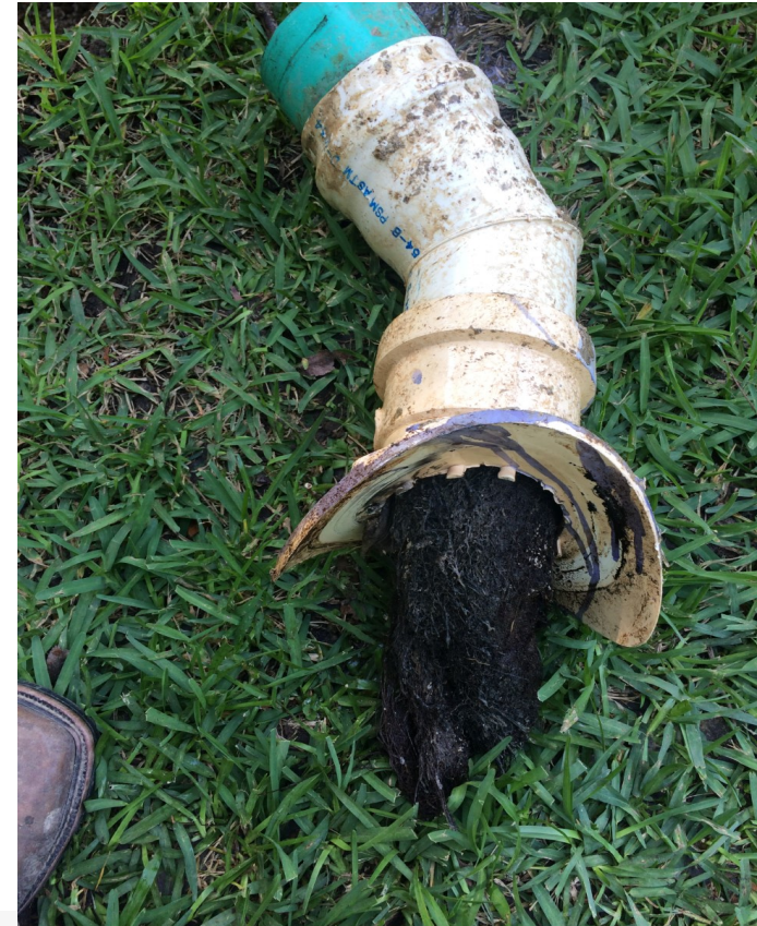
Sewer Line with Tree Roots
