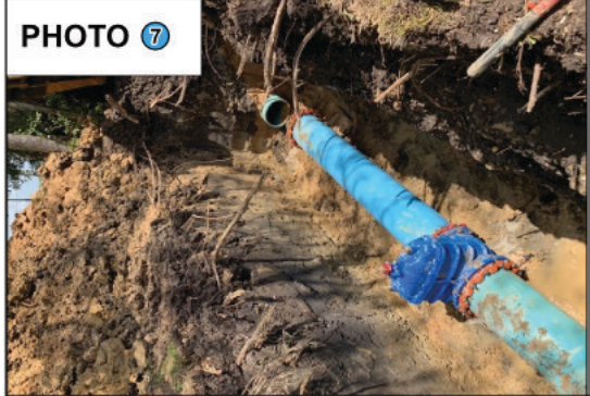
PHOTO 7 Water Line Valve Problem: Water line valves are aging and need to be evaluated. Solution: Valve survey and replacement program.
