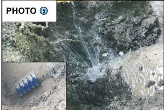
PHOTO 5 Water Distribution Main Line Problem: Water Main break due to aging distribution line. Solution: Water System Rehabilitation.
