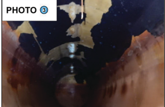
PHOTO 3 Hydro Tank Problem: 80% of interior coating has deteriorated over time, and metal is beginning to corrode. Solution: Replace Hydro Tank due to severity of the conditions.
