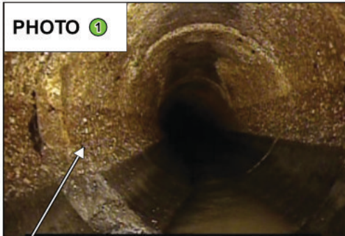
PHOTO 1 Problem: Broken 24" Reinforced Concrete Pipe at Joint. Solution: Pipeburst Method. Newport Section 1
