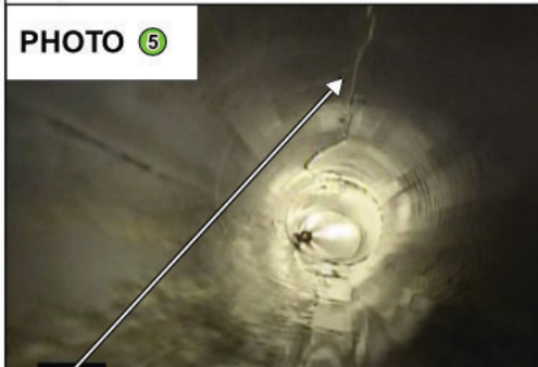
PHOTO 5 Problem: Longitudinal Crack at top of 12" Truss Pipe. Solution: Pipeburst Method. Newport Section 2 and Oaks at Newport Section 1
