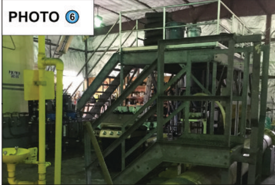
PHOTO 6 Surface Water Treatment Plant Problem: The space and access is limited. Solution: Improve and maximize space during Plant Expansion.
