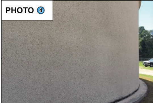
PHOTO 4 Ground Storage Tank Problem: Ground Storage Tank coating is deteriorating on exterior. Solution: Recoating of exterior surface.
