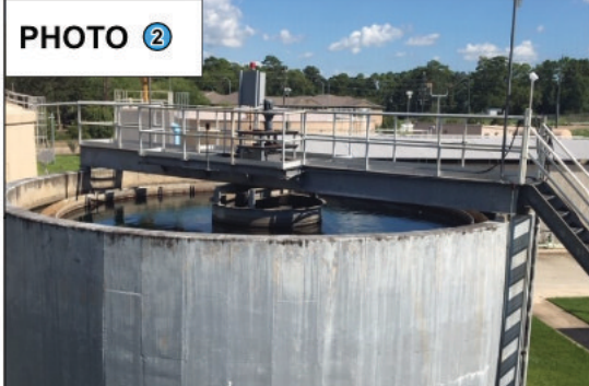
PHOTO 2 Surface Water Treatment Plant Clarifier Problem: Tonka Clarifier is not working properly and is now out of service. Solution: Repair Clarifier before further damage occurs.
