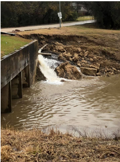
Main Line Break on Wherry Dr. prior to repair
